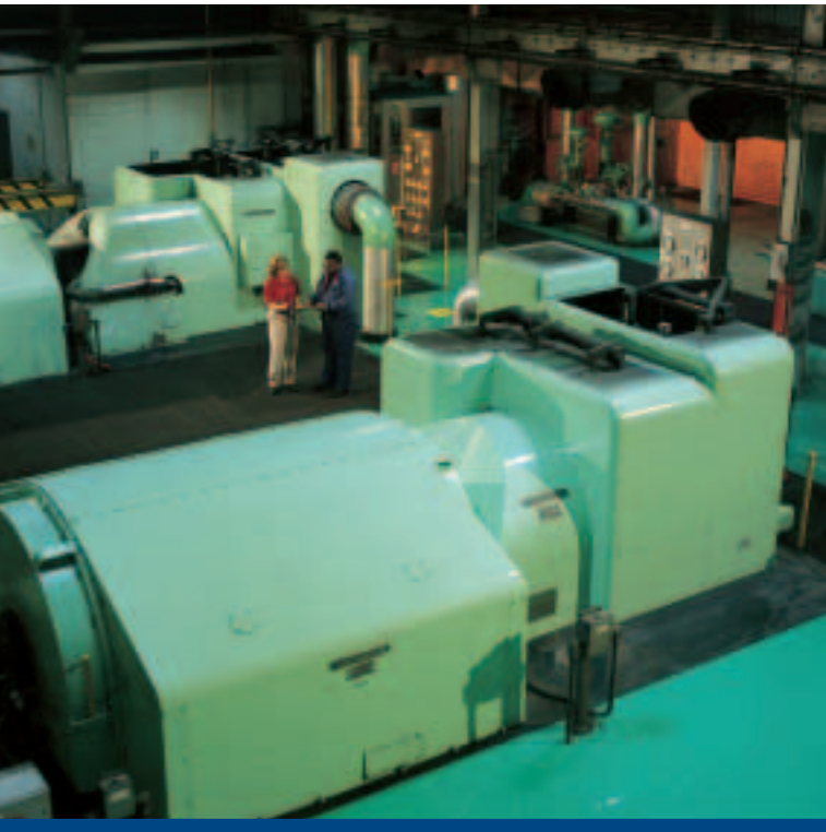
Valdosta Turbine Room
